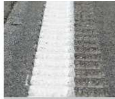
Example of an edge line rumble stripe.
